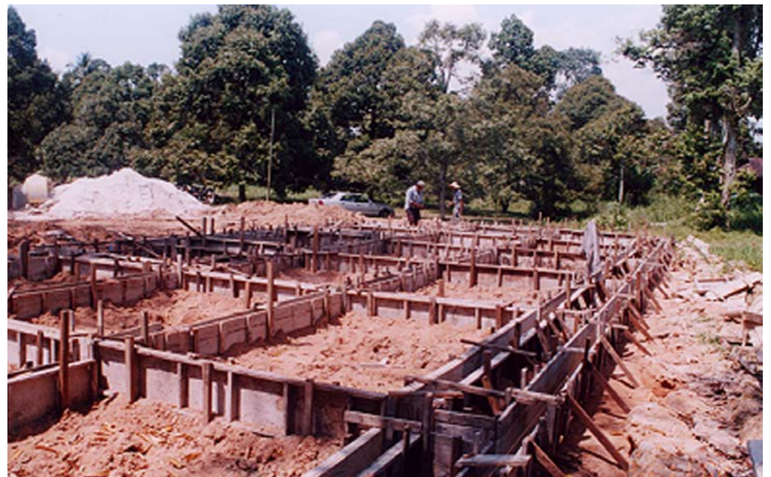
This is followed by the process of preparation and casting of the ground beams
