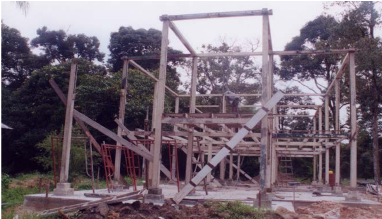
pictures shows the almost completed main structural timber framework prior to the installation of roof girders and trusses
